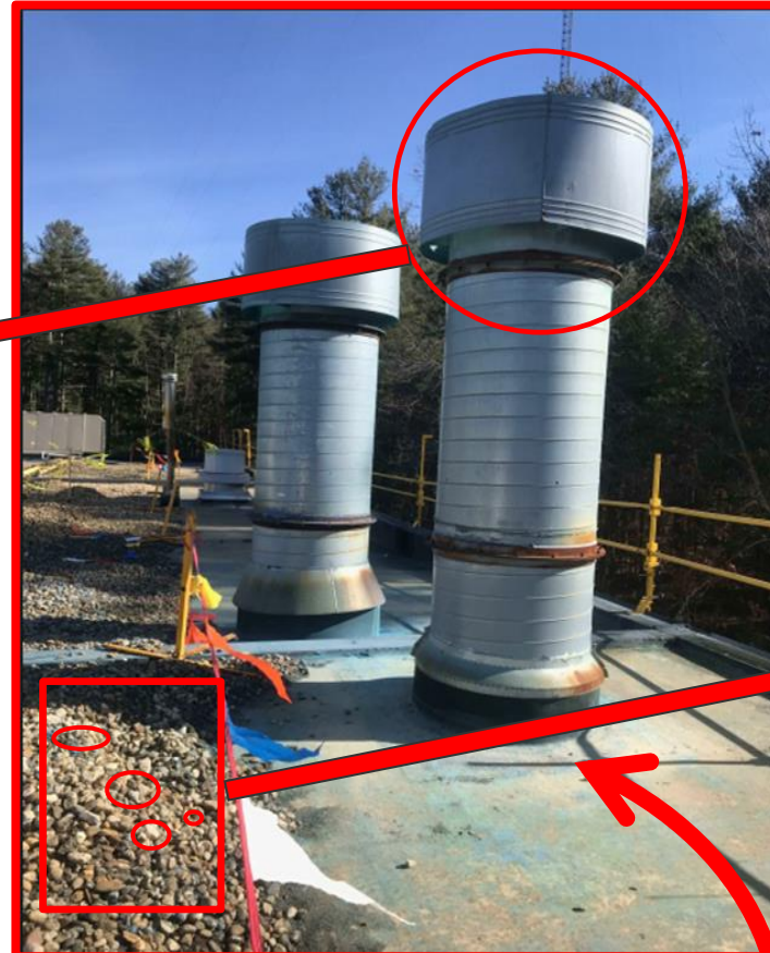
Roof Ballast and Roof Stack Residue Under Roof Ballast
