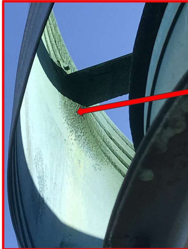
Coating Agglomeration on Inside of Stack Cap ≤17,200,000 ng/Kg PFOA
