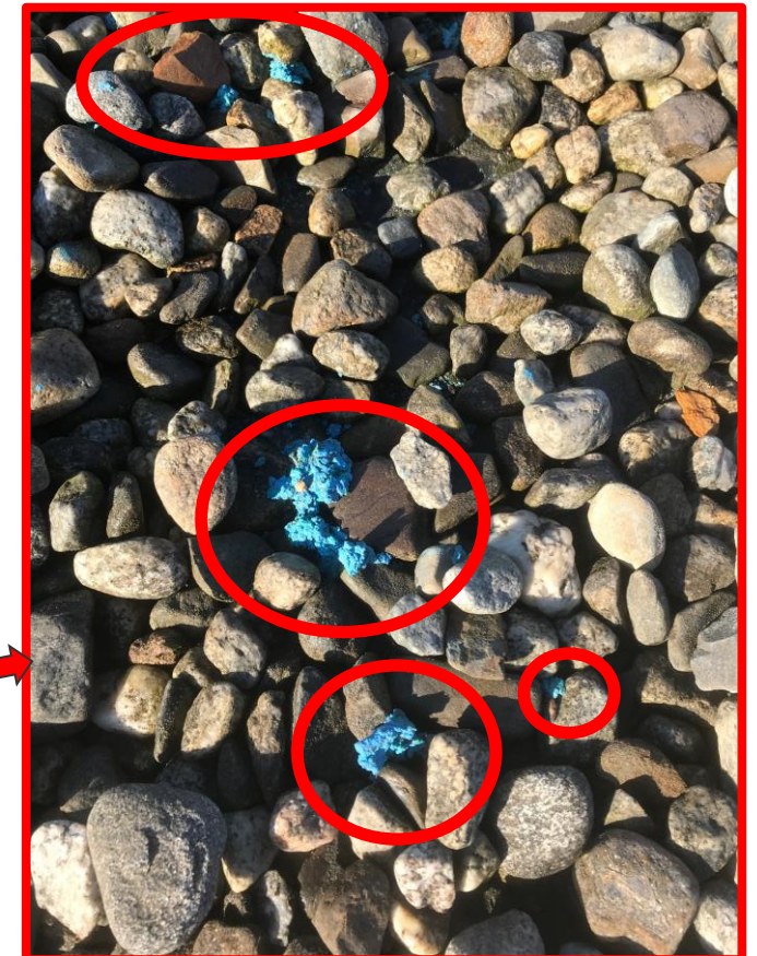
PFAS Residue in Roof Ballast from Chunking of Coating Agglomeration Occurring in Stacks ≤13,000,000 ng/Kg PFOA
