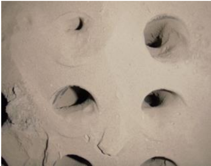
Tubular Primary Air Heater
