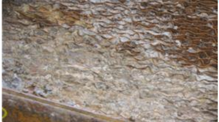
Rotary Air Preheater Basket Fouling
